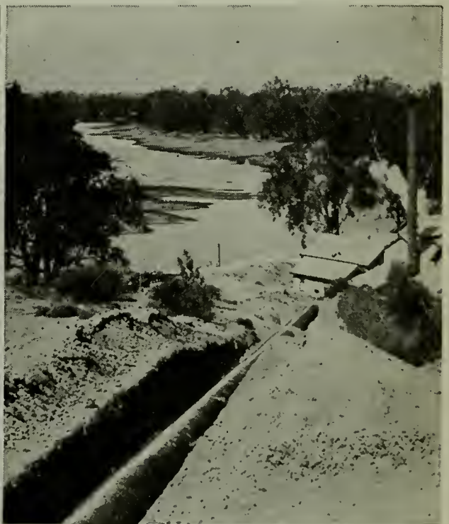
Here we see a pumping station in Australia.
